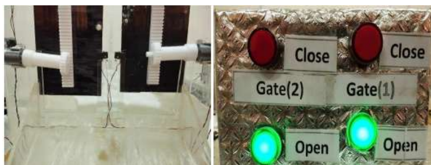
Figure 26: Both gates are opened, and the indicating lamps are on.
